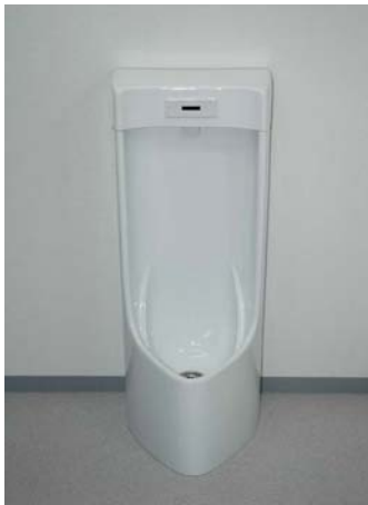
Figure 1. Water recycling urinal.
