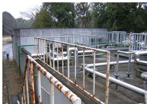
Figure 8. Domestic wastewater treatment facility in Minori service area.
