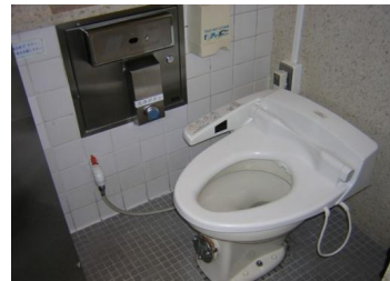
Fig. 6: Existed toilet in Moriya service area
