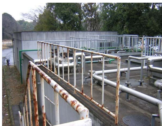
Figure 8. Domestic wastewater treatment facility in Minori service area.
