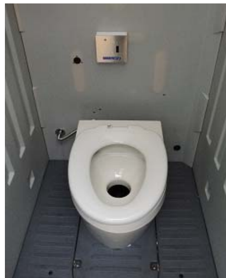
Figure 2. Water recycling urine-diverting toilet.
