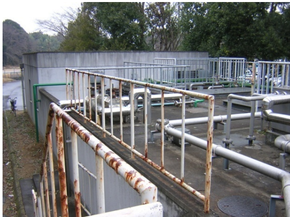
Figure 6, Domestic wastewater treatment facility in Minori Parking Area
