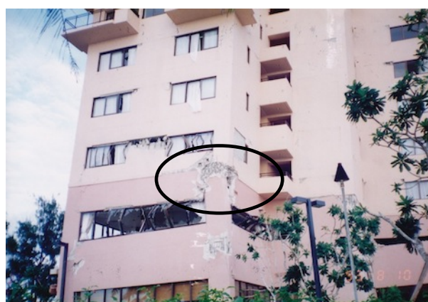
Figure 2: Failure of corner beam-column joint in Guam Island Earthquake in 1993.
