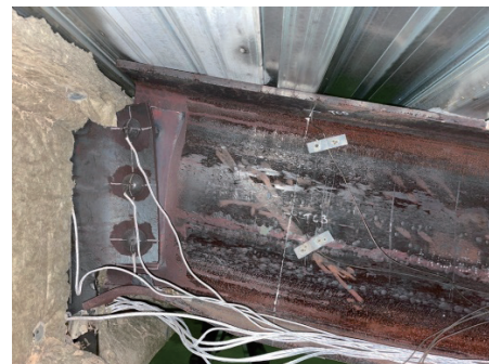
Photo 4 Deformed connection observed after experiment
