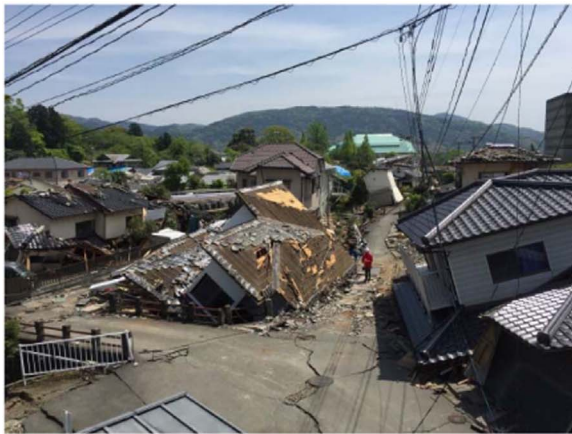
(a) Collapsed wooden houses
