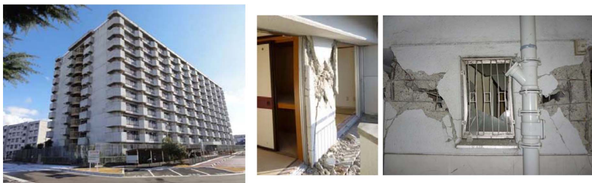
(a) Non-structural walls failed in shear
