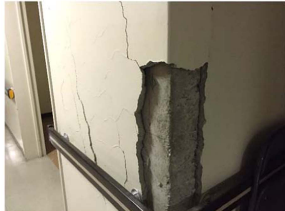
(b) Minor cracks on columns
