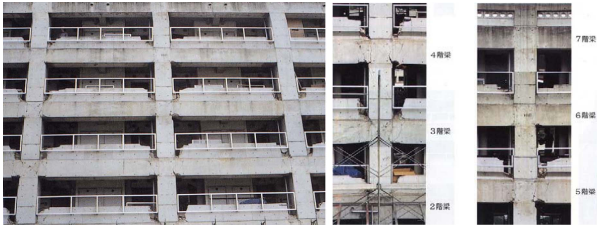
(a) Flexural cracks of beams
